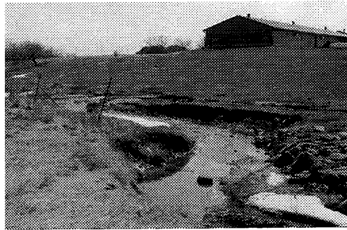
Photo 5: Erosion and bank instability due to a lack of vegetation (April 1993).
